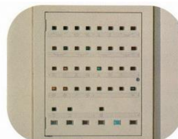
Picture 52 – Comprehensive alarm systems for air conditions, pumps, lifts, sprinklers, and ventilation systems
